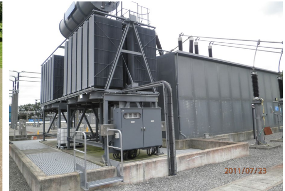
400 kV Power Transformer
