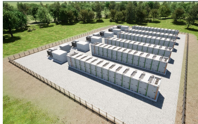
Battery Storage Compound
